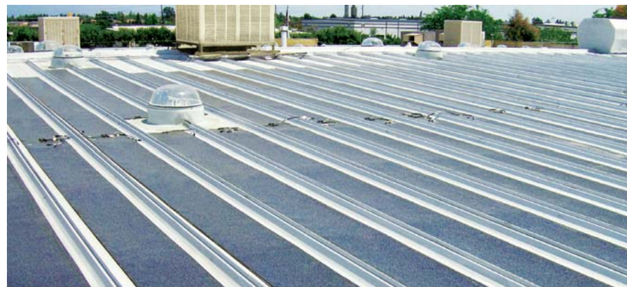
Kawneer's Visalia, California manufacturing facility serves as the host for DEERS Solution™, a patent-pending solar rooftop attachment system developed by DEERS. The system is owned and operated by Constellation Energy Projects & Services. The 588,000-watt Photovoltaic (PV)
